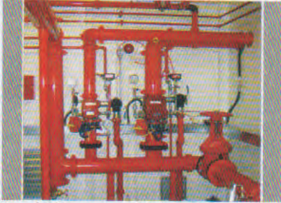
Fire fighting pipes/Hydrant
